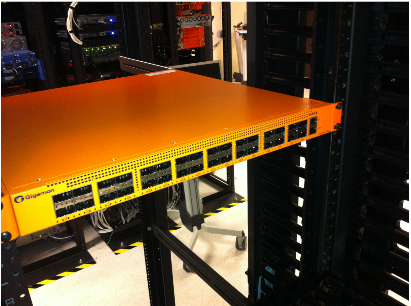
Figure 6 Front View of the Mounted Node to the Four-Post Rack
